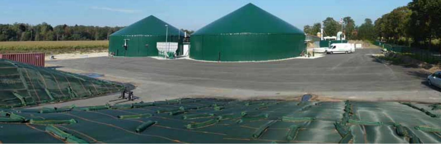
Biogasanlage in Raming, Geeste
